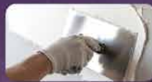
Apply Mobi Fine Filler Apply 2 Coats, Sand the wall and dust it off
